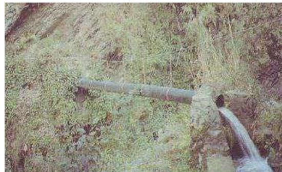
फोटो : Pipe crossing over natural stream, Source SSIM
