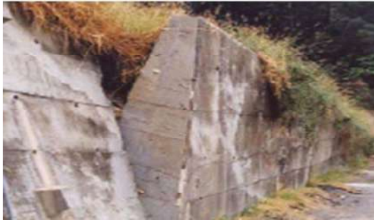
फोटो : Shifting of Concrete Retaining Wall due to excess surcharged load on backfill
