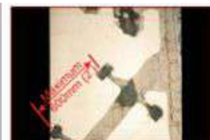
Hammer in 'C' clamp at maximum distance of 900mm in the mortar joint perpendicular to the crack.
