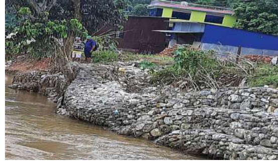
फोटो : Failure of Gabion Wall due to river bank scouring and poor construction method adopted, Damauli.
