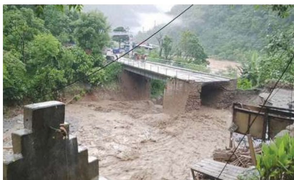
फोटो : Scouring of Abutment backfilling (More coarse grained material) due to peak Flood in Mouwakhola, Dhanding, Source: Online news
