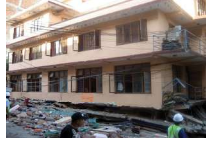
फोटो : Soft Storey Failure from Earthquake
