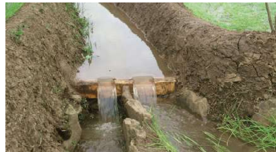
फोटो : Reduction on canal capacity due to growth of vegetation at side slopes and even siltation in bed.
