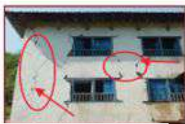
Grade 3 cracks in plastered walls
