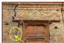
Grade 3 cracks in unplastered walls
