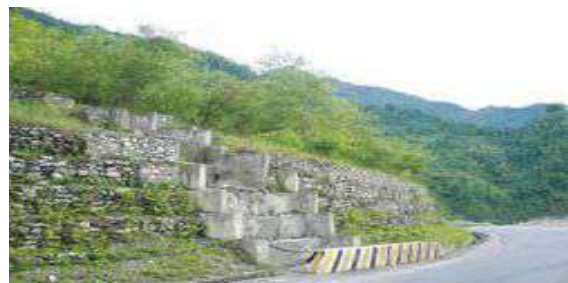
फोटो : Krishnavir Landslide before treatment
